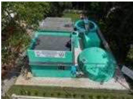
360 KLD STP at General Hospital, Thrissur
