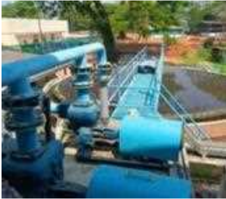
500 KLD STP at Kozhikode medical College
