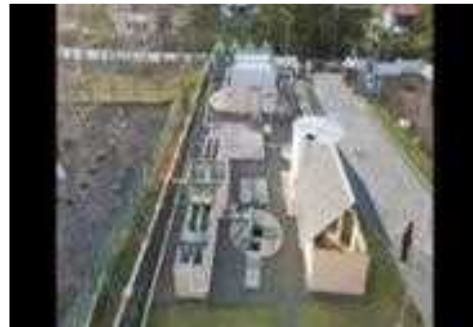
1 MLD CSTP at Padanappalam, Kannur
